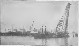
The mighty pile driver "Aruba" juts 105 feet above the harbor as it prepares to drive another pile. Its hammer weighs ten tons and operates on steam power.
